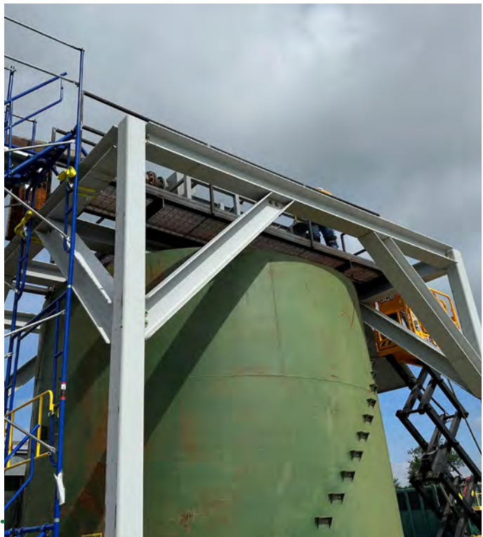
Elm Fork - Mixing Tank and Shaker Screen
